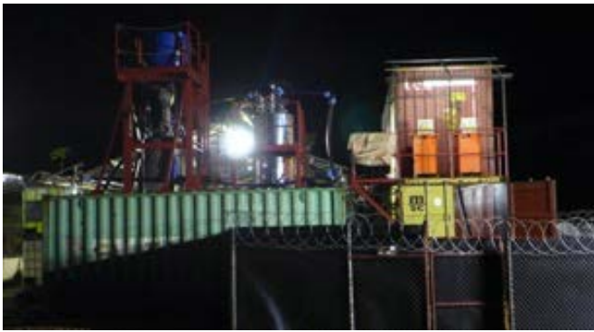
Rectifiers being commissioned
